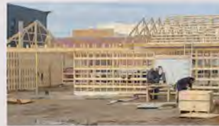
Grass Roots New Building is going up after the demolition of Derelict Properties
